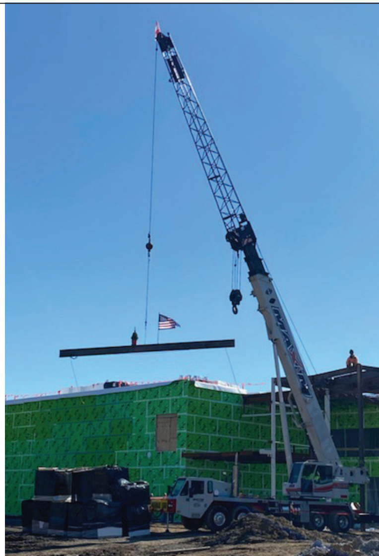
The Topping Off Ceremony – The last beam was placed in the superstructure in February.
